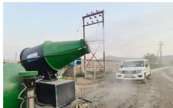
Fog Cannon Dust suppression system in Ash Dyke
