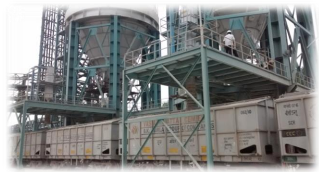
Dry Ash supply Rake Loading System
